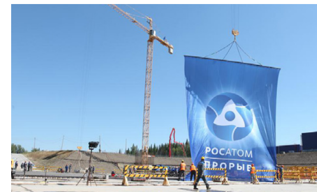
The PDEF is being built as part of ROSATOM’s strategic project code-named Proryv (‘Breakthrough’), which is focused on creating a new technological platform for the nuclear power industry. It involves the widespread adoption of technologies for the recycling of nuclear materials. This will considerably increase the availability of feedstock for the nuclear power industry and will help to address the issue of spent nuclear fuel and radioactive waste accumulation by reusing SNF reprocessing products instead of storing them and by drastically reducing the volume and radioactivity of waste.
